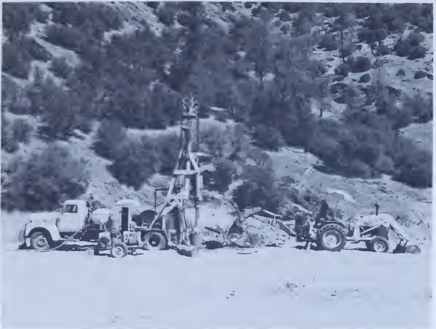
Figure 39.—Clamshell excavator and backhoe unit with reverse shovel exploring the gravel bars at Auburn Dam, California. P1859-245-5533.
